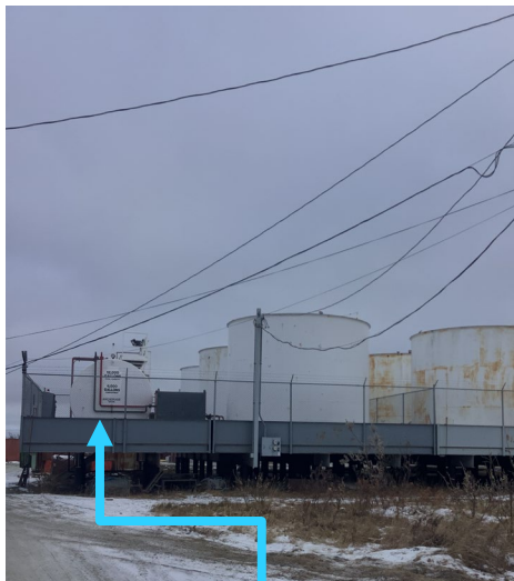
Improper routing of electrical lines through tank farm corners.
