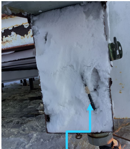
Snow packed into the main power feed for the bulk fuel farm.
