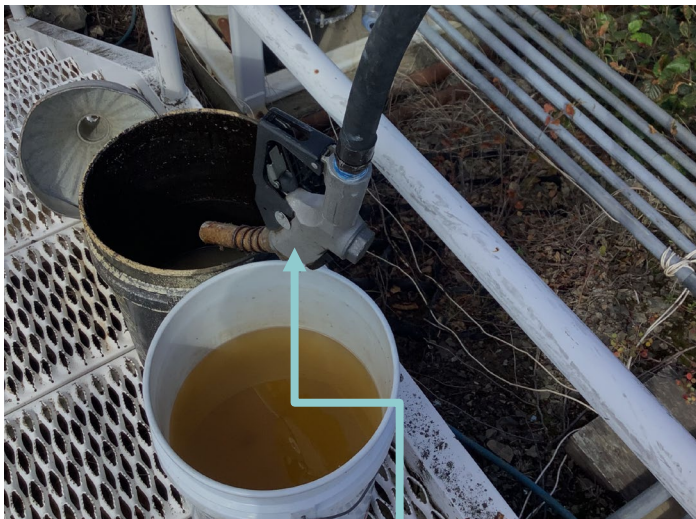
Leaky fuel nozzle draining into an open-top bucket.
