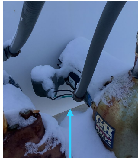
Improper wiring protection near highly flammable fluid storage.
