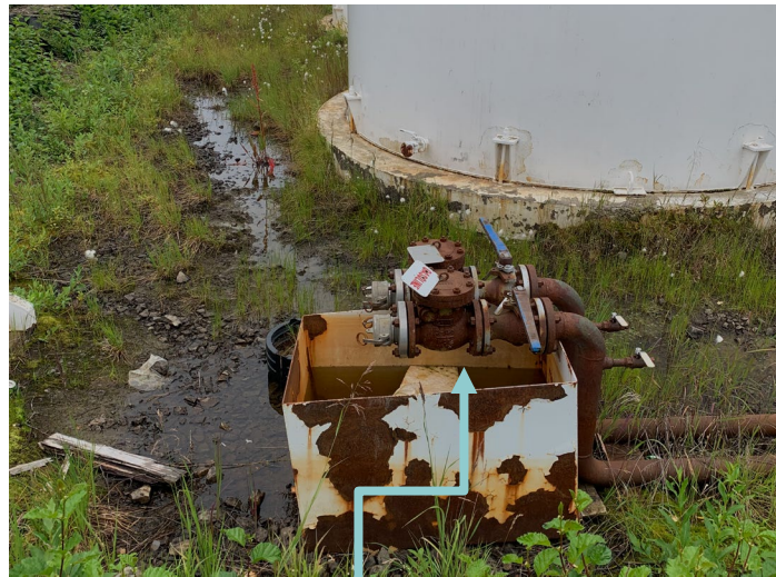
Containment is filled with water and trash, leading to untreated contaminated water poured onto the ground.
