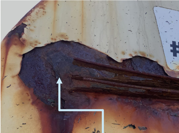
Deep corrosion poses a risk of tank shell failure.
